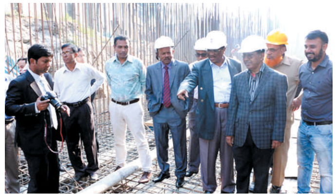
Chairman and Member of BOT, Vice Chancellor, Treasurer, Registrar along with others visiting the construction progress at the Mazar Road in February 2016
